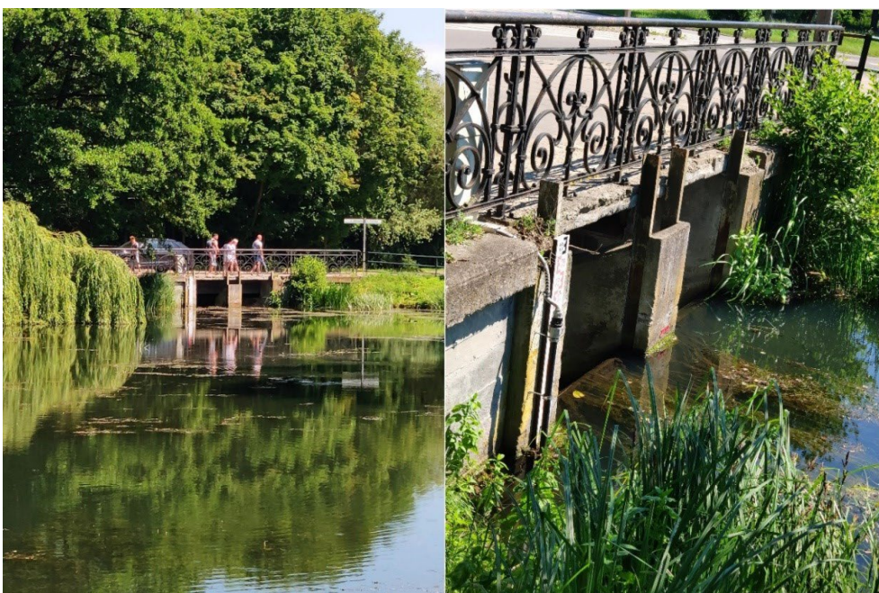
Figure 1.9. The cross-section shown on Figure 1.7 where students measured the load of the overflow with a sharp edge (weir).
